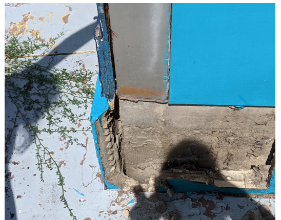
MISSING TERRACOTTA BASE
