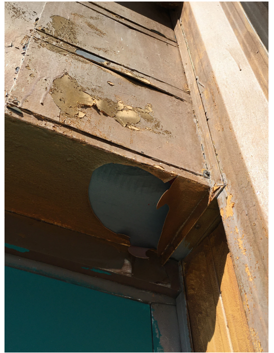
LAYERS OF PAINT FLAKING OFF
