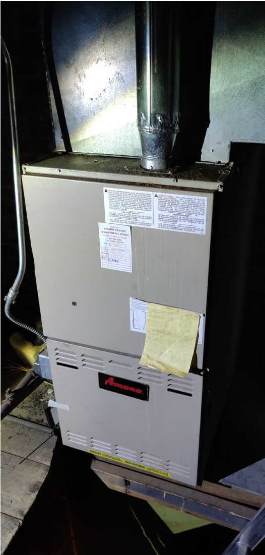
EXISTING MECHANICAL SYSTEM
