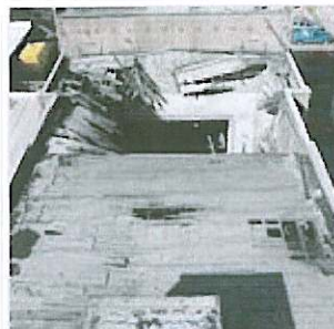
The Fox Theater roof demolition begins Sunday. People are advised to stay a safe distance away. Boomerang file photo
